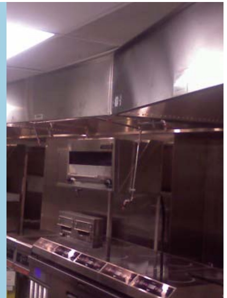
Unique installation of Capture Jet® hoods due to structure of the CN Towers circular pod.
